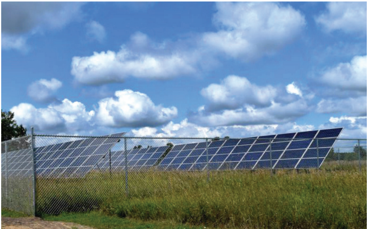
One of five solar arrays that make up the Band's Community Solar Garden
