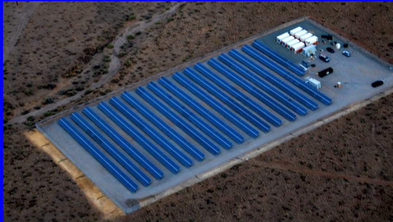
2011, NM: 500kW, 2.5MWh with PV
