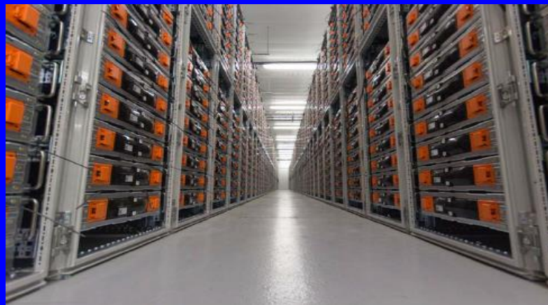
2014, CA: 8MW / 32MWh Wind Ramps
