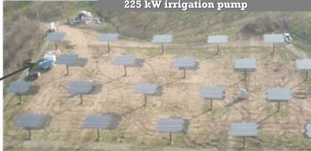
2 axis tracking PV system
