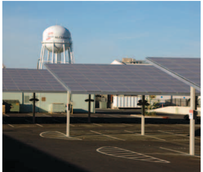
Sacramento Municipal Utility District's Feed-in Tariff Program
