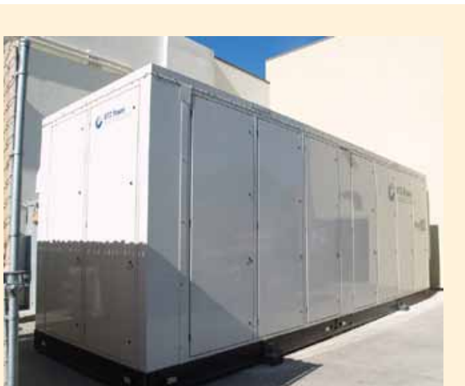
The fuel cell at an Albertsons supermarket in San Diego.
