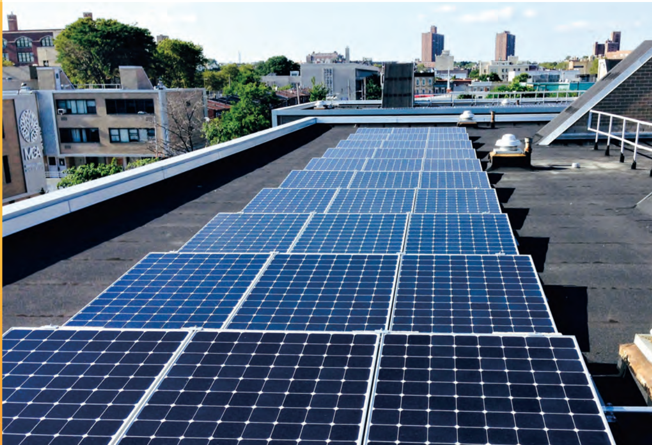
Marcus Garvey Village solar array, courtesy of L+M Development Partners Inc.
