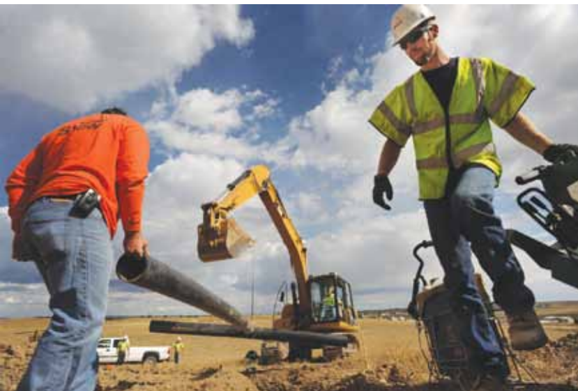
Chris Roma, left, and Danny Smith, right, of Shaw Environmental construct a piping system to extract methane gas from the Larimer County Landfill. The methane gas will be converted to electricity and represents the first clean energy project partially funded by the Colorado Carbon Fund.
